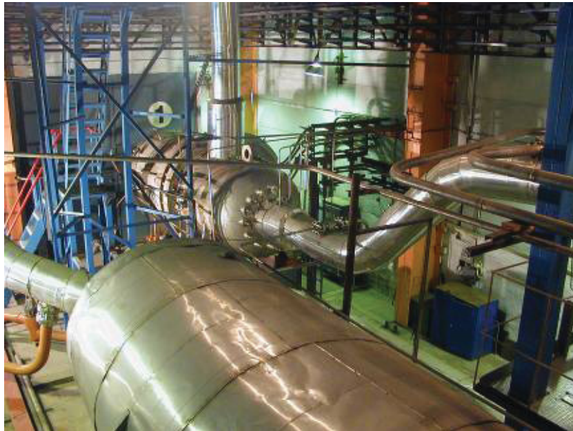
Figure 3-1. High-Temperature Helium Facility for Heat-Exchange Equipment Tests
