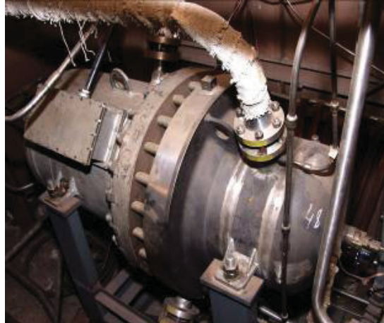
Figure 3-9. Gas circulator for the Multipurpose Research Complex
