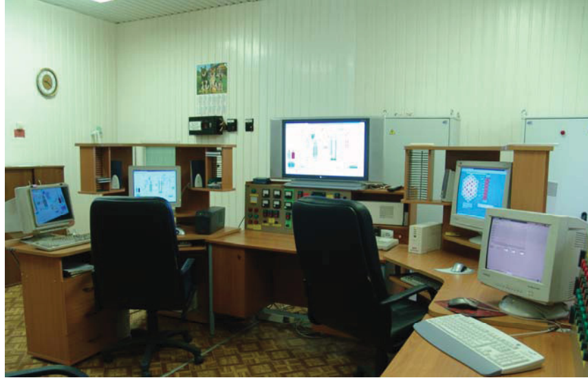
Figure 3-28. Control Room of PARAMETER Test Facility at NPO Lutch
