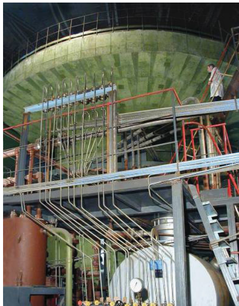
Figure 3-14. Main Circulator Test Facility
